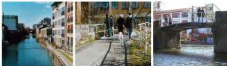
Three views of Kingsland Basin footbridge showing the route of six NG 400kV cables beneath the towpath of Regents Canal, London
